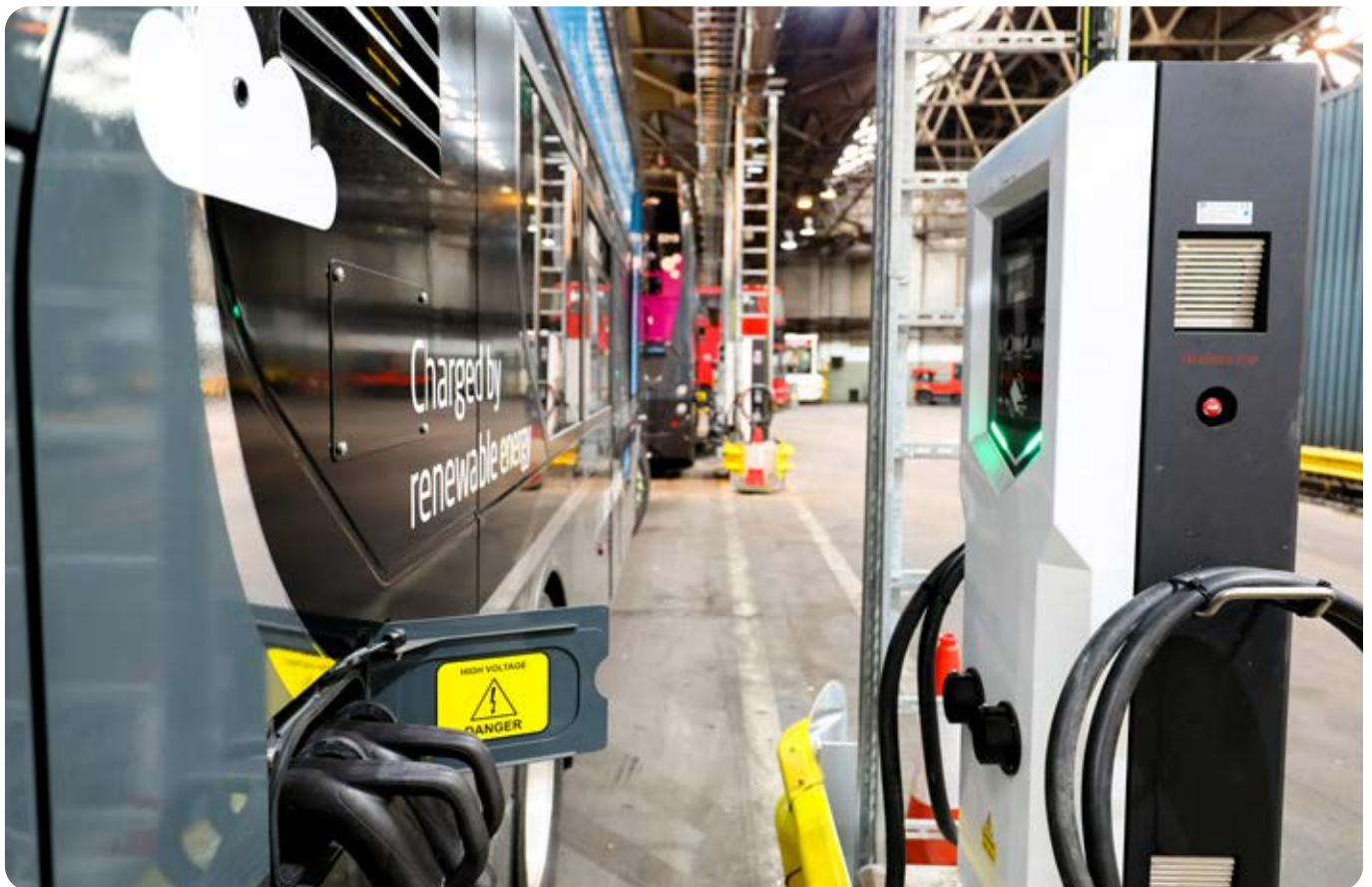
Charging station, National Express Electric Bus 900
